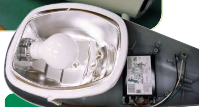
Cobra head for street lighting. 100 watt HPS retro-fitted to a 55 watt Induction lighting system with Profile ballast
